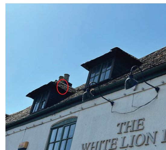
Photo 5 B1- Dormer windows with Lifted tiles
