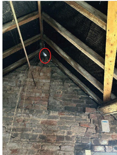
Photo 9: B2 - with a gap in the lining of the loft of the southern gable end elevation
