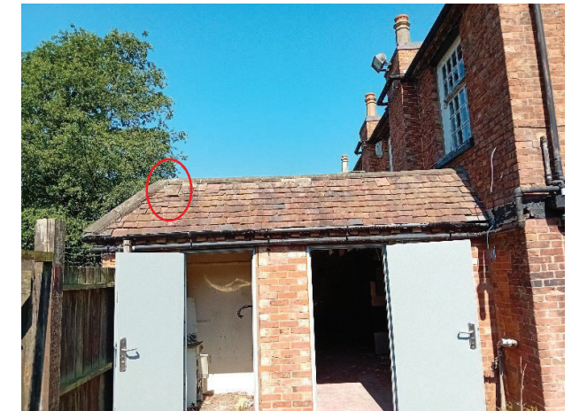
Photo 2: B1 - Eastern Elevation ground floor roof with lifted tile
