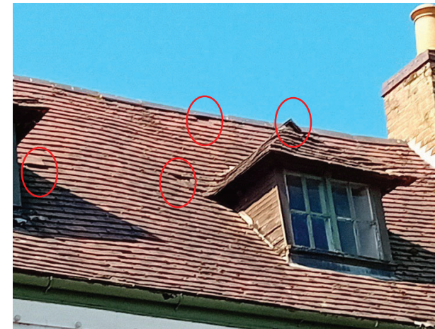
Photo 1: B1 - Northern Elevation with missing and lifted tiles
