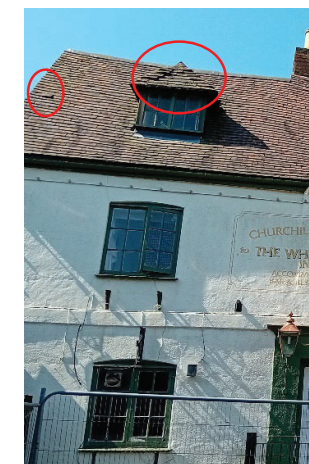
Photo 4: B1 - Northern elevation with dormer window showing lifted tiles
