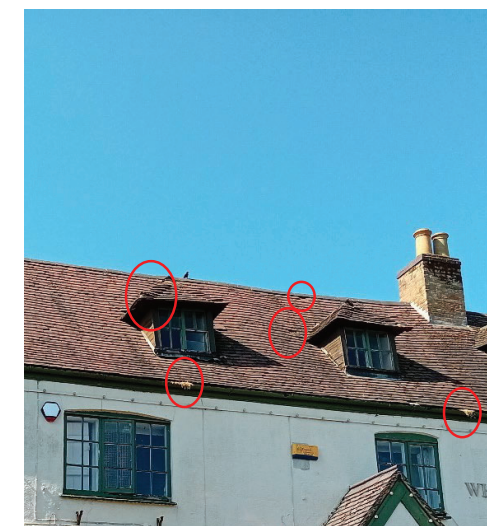
Photo 6: B1 - Northern elevation showing lifted and missing tiles around the dormer windows and disused bird nests within the guttering.
