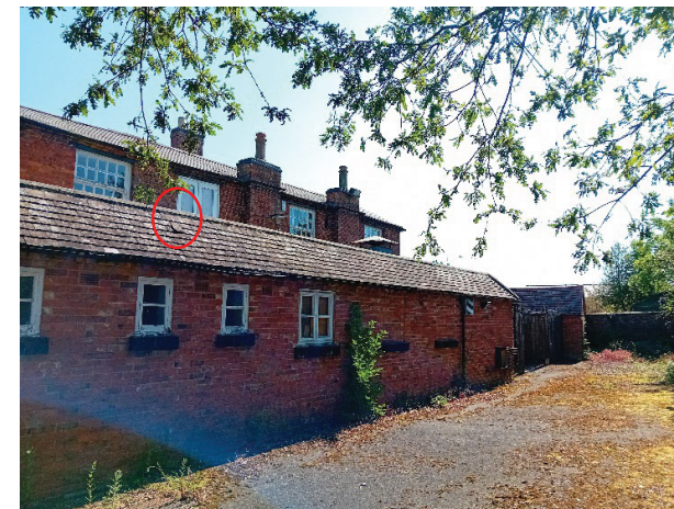
Photo 3: B1 - Southern elevation with lifted tile
