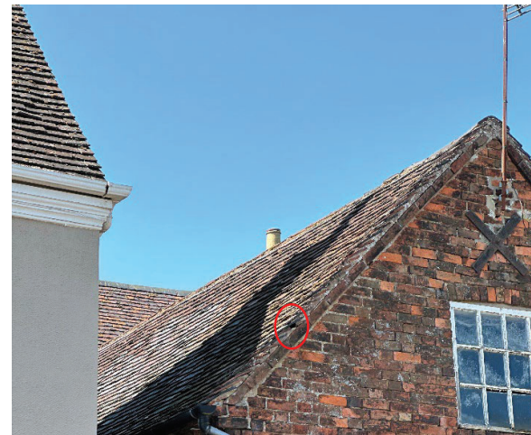
Photo 10: B2 Northern elevation with missing tiles
